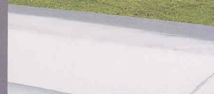
One-year-old Winnebago Industries' fiberglass roof
